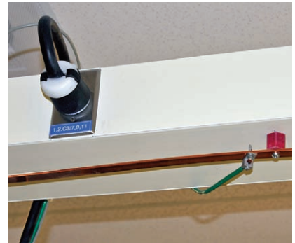
FIGURE 2. Ground bars, located under electrical wiring conduits, provide access to earth ground that is located deep under the lab. The grounding system has lowered power-line noise in the new lab. Courtesy of Northrop Grumman.
